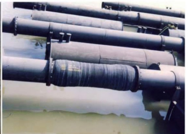
Discharge Hose in water pipe line at Kashmir, INDIA
