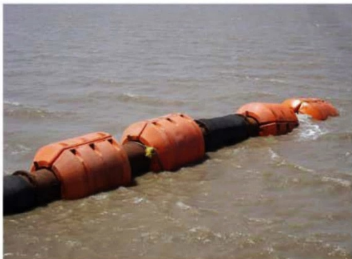
Discharge Line Along with Floaters
